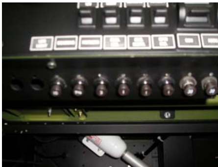
Picture: Circuit breakers under the instrument panel
